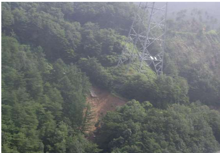
Fig. 2 Actual case of a slope and foundation failure (KEPCO, 2013)
