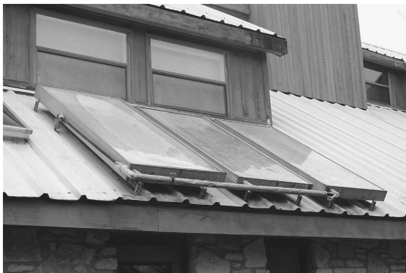
Fig. 2. Exterior view of collector panel arrangement.
